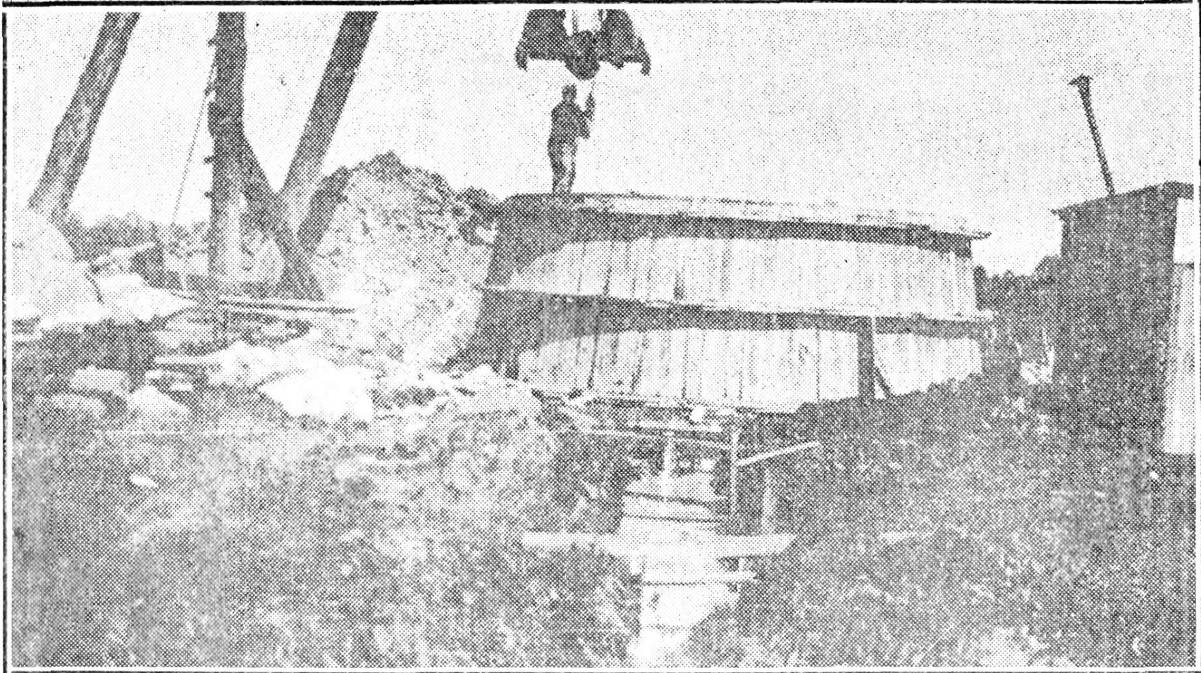
Sixteen foot well under construction. Excavating clay from inside of well casing.. Concrete in place but forms not yet removed.
